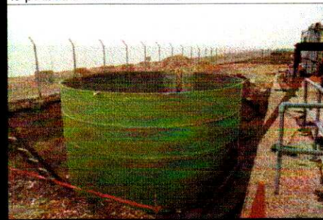
8. The Fiberloc joint is placed in position and sealed. The tank is then made level and concrete is poured to lock the tank down.
