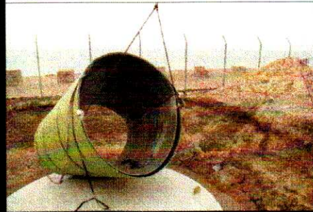
5. The strap positions of the crane are changed to allow the tank to be 'stood up' in the centre of the slab.
