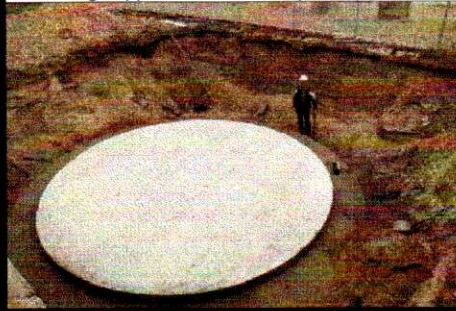
2. A circular, concrete base has already been prepared for the 'Fiberloc Tank', using GRP shuttering supplied in advance by Camplas.
